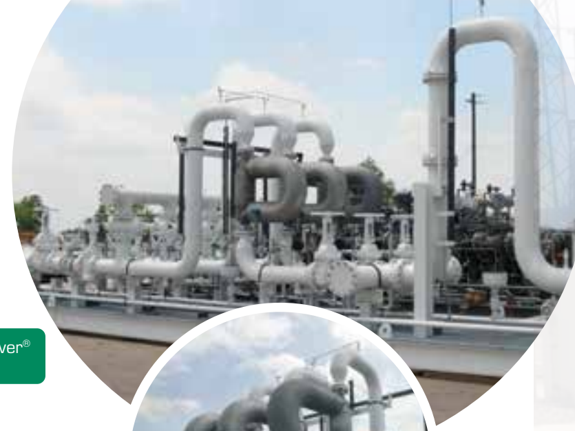
Three run 4" ANSI 150 coriolis metering system for West Texas.
