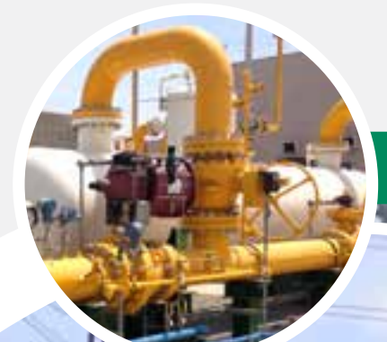
City Gate Station
